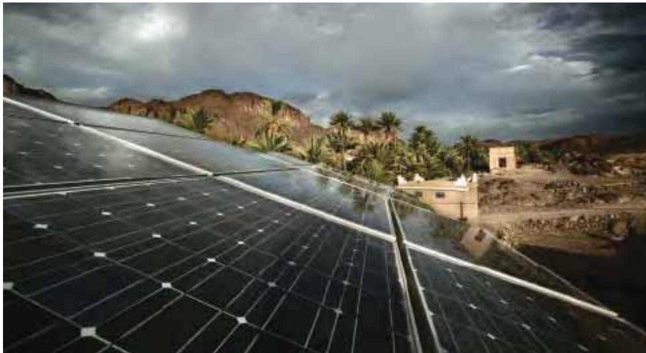
▲ Isofoton photovoltaic micro-plants in Morocco. The region has one of the highest potentials for renewable energy in the world. ©Isofoton.es. Licensed under the Creative Commons Attribution 3.0 Unported license.
