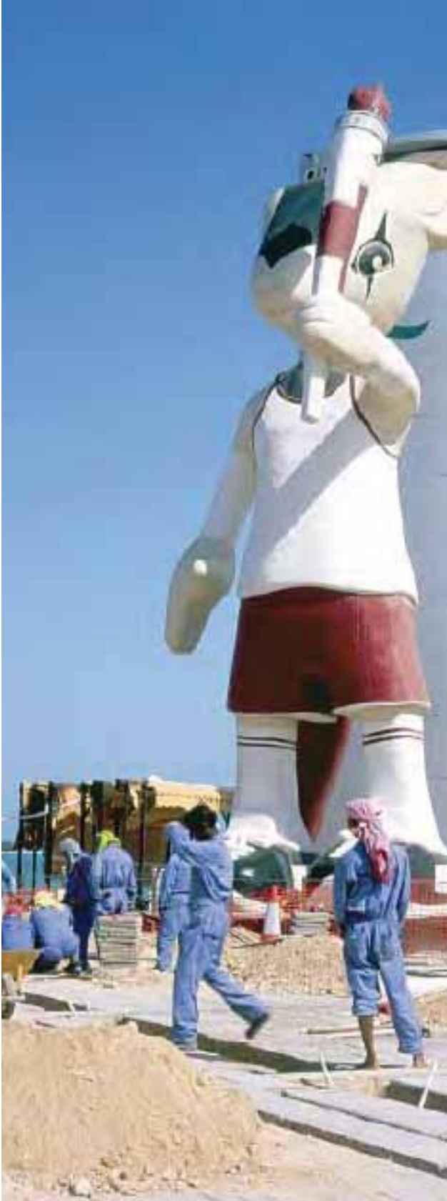
▲ Doha, Qatar. Asian labourers at work on the drainage system in front of Qatar's national "Orry the Oryx" mascot, originally created for the 2006 Asian Games. Qatar's impressive infrastructure is being created by a vast army of cheap labourers drawn from across Asia. ©Paul Cowan/iStockphoto
