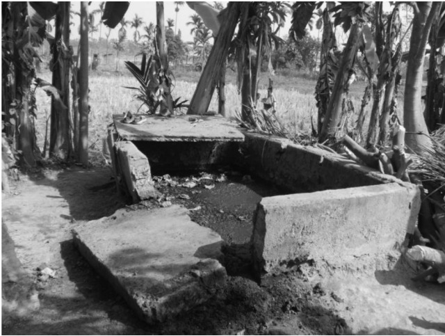
Fig. 2. Non-functional biogas unit at household number 12 (see Table 1) which has not been repaired for 6 months.
